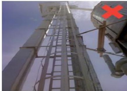
No ladders > 7.3 m
