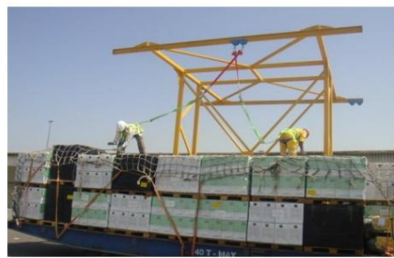
Tarpaulin platform - External
