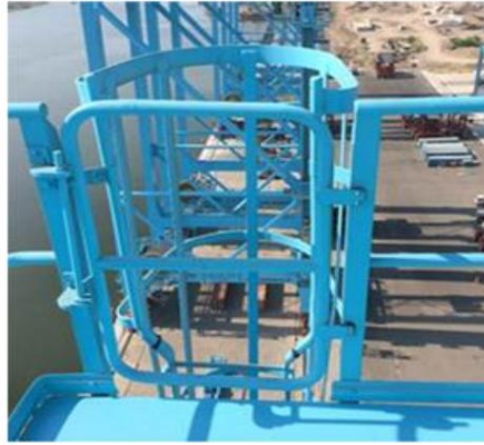
Ladders with a folding gate to avoid fall from the platform
